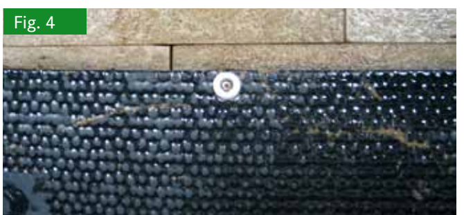
Fig. 4 Fastening of the mat with hard rubber edge to the elements of slatted floor below
