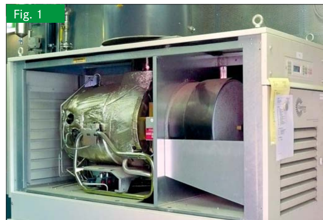
Microgasturbine Capstone CR 65. Photo: Bekker
