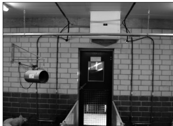
Fig. 1: Directing intake air through feed passage doors, and removing it through extraction points near the inlets, heating with gas canons
