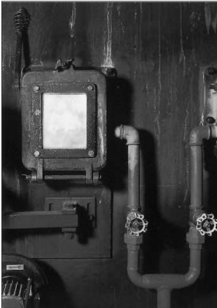
Fig. 1: Fuel burns almost completely in the biomass boiler. Ash proportion is around 1%.
