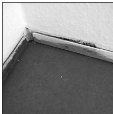
Fig. 2: Mould fungi behind the base board in the living area
