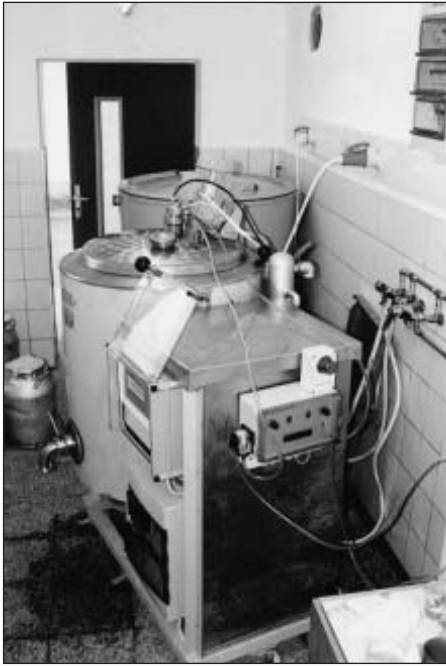
Fig. 2: Production plant installed in Niederschöna cooperative farm
